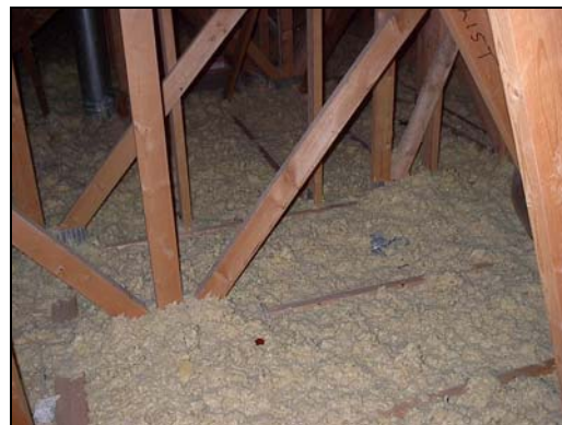
Inadequate levels of insulation
