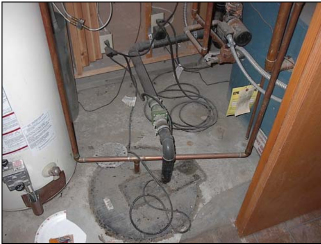
Sealed sump system in mechanical room
