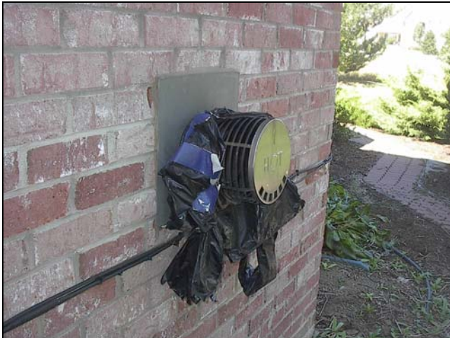
Chimney cover requires removal during use of fireplace
