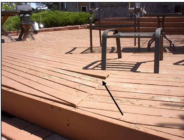
Deck requires sealant and repair to deck boards (trip hazard)
