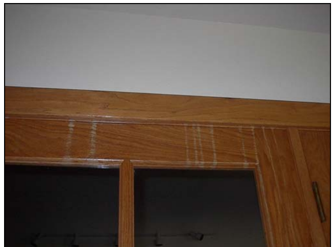
Discoloration on door entering sun room
