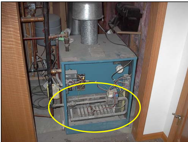
Burners require regular maintenance
