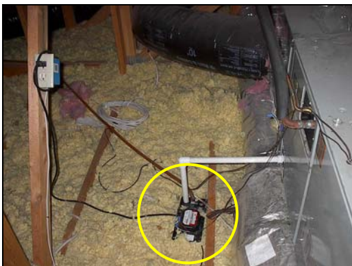
Sump pump at A/C unit
