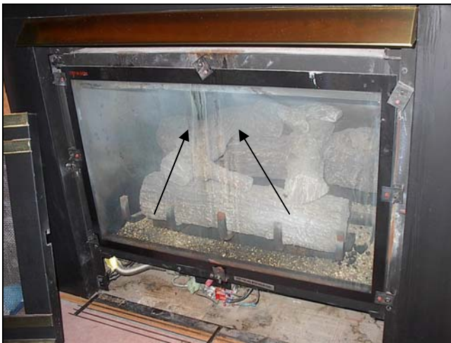
Evidence of oxidation
