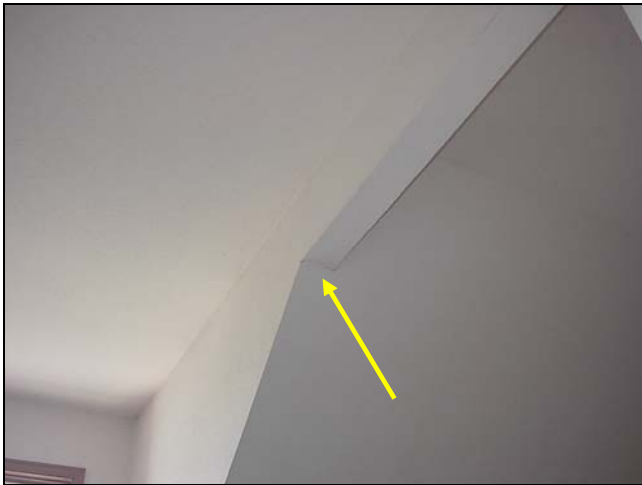
Crack in living room ceiling / wall intersection
