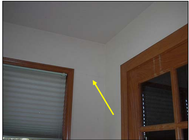
Crack in sun room wall
