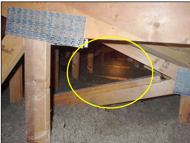
Levels of insulation less than adequate above Bdrm. 2
