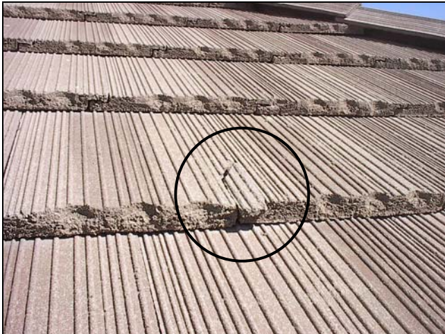
Damaged roof tile
