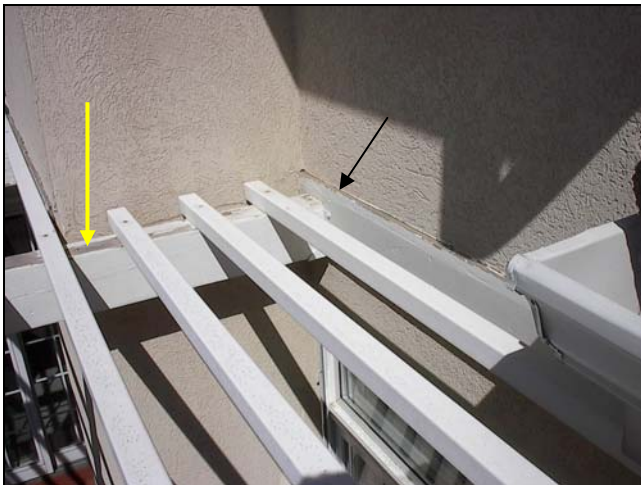
Sealant required at stucco and wood ledger Peeling paint and exposed wood (yellow arrow)
