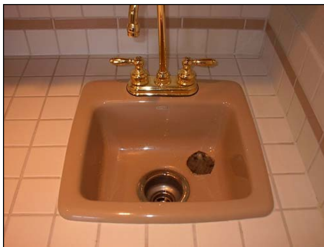
Damaged sink in wet bar
