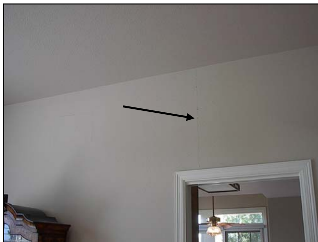
Crack in dining room wall
