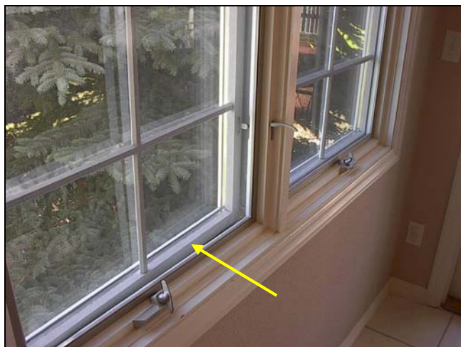
Peeling paint at window frames
