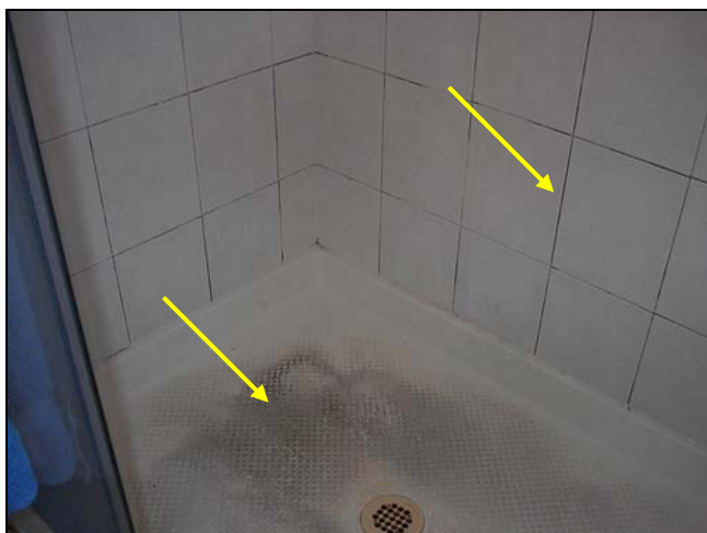
Discoloration of shower floor and grout
