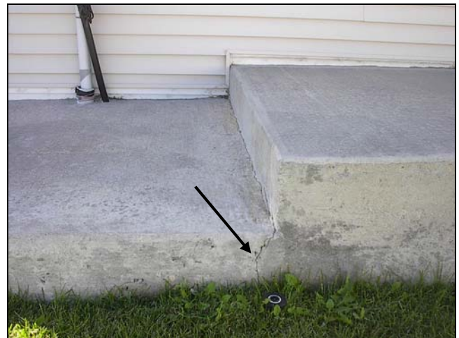
Crack at front walkway
