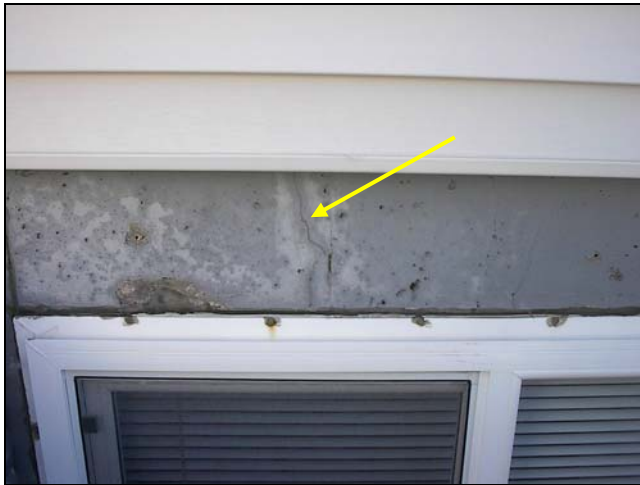
Cracking is evident in concrete foundation wall
