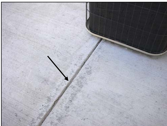
Crack in control joint at rear patio
