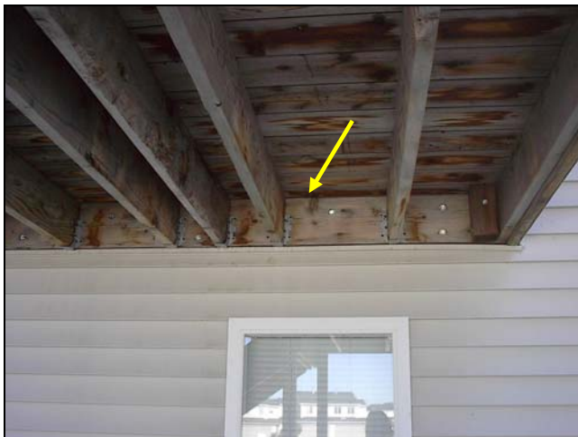
Flashing not evident at ledgerboard
