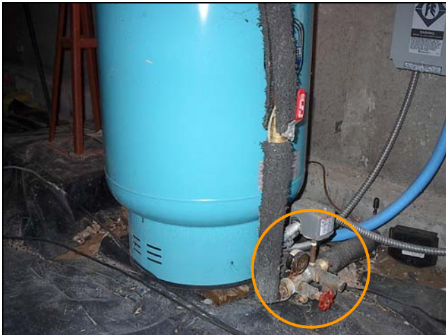
Rust is evident
