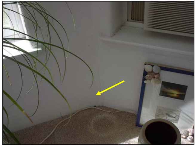
Cracking in Bedroom 1
