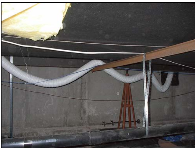
Dryer duct has a negative slope
