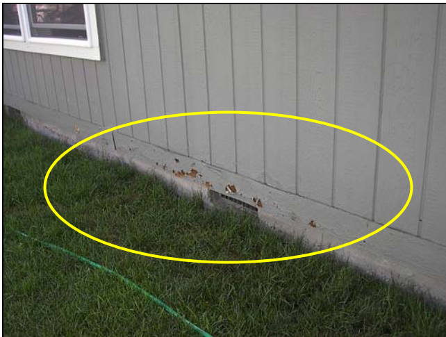
Evidence of water absorption and damage
