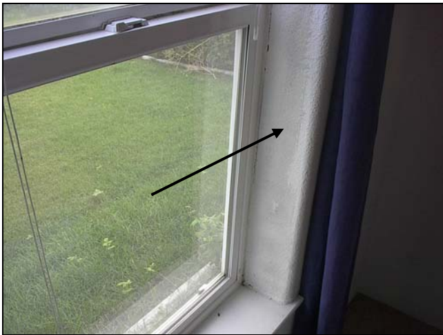
Discoloration suggests water intrusion at window
