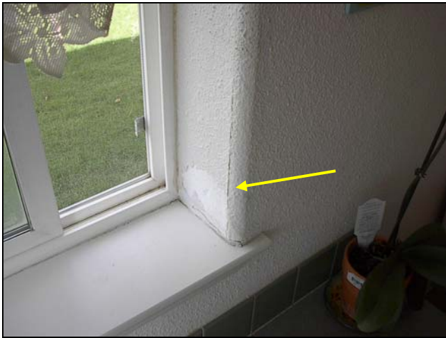
Cracking evident in Bath 1
