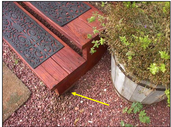
Wood in contact with soil at front step
