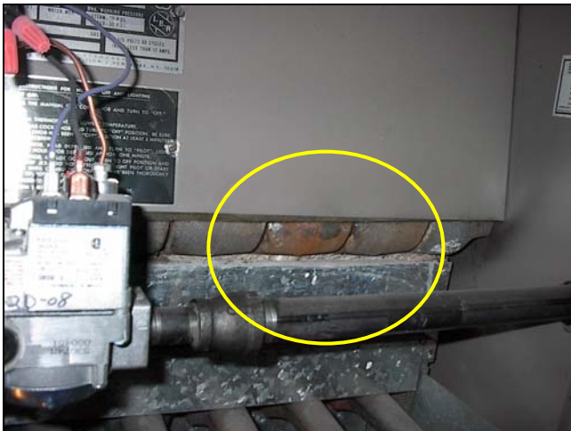
Rust near heat exchanger of boiler
