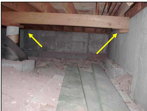
Bearing in beam pocket and shims are suspect
