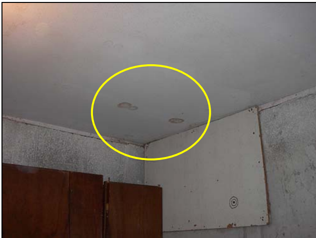
Elevated moisture content at these watermarks
