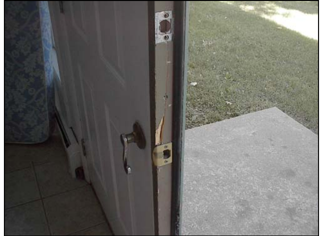
Damaged front entrance door
