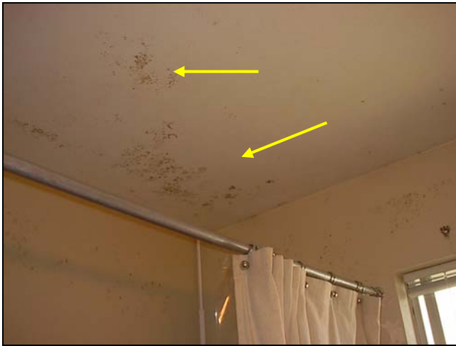
Mold-like stains on Unit C bathroom ceiling
