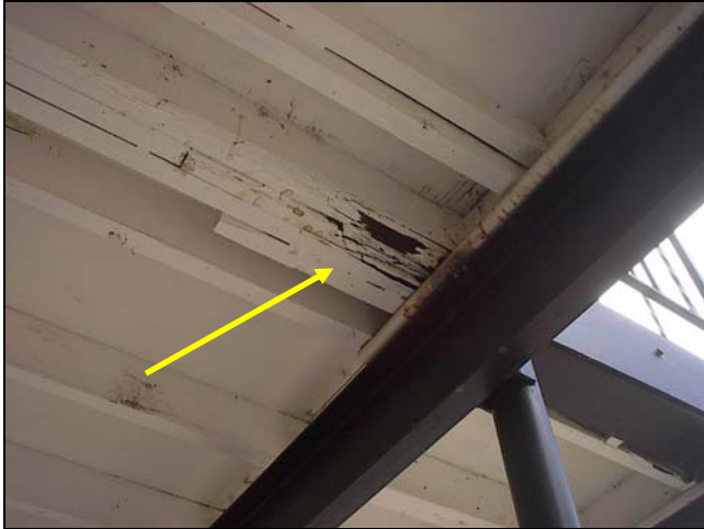
Balcony joists are water damaged
