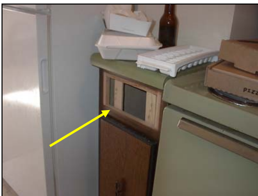
Damaged kitchen cabinet face – Unit #C-201
