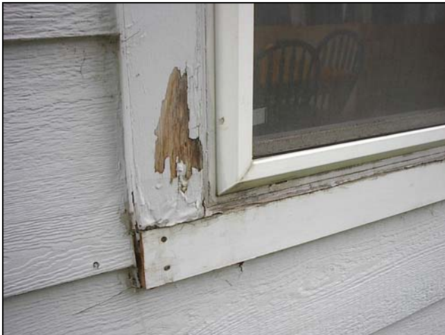
Water damaged wood window frame
