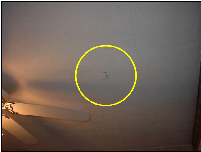
Blistering paint in kitchen ceiling
