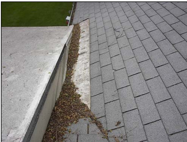
Debris in roof valley of dissimilar surfaces
