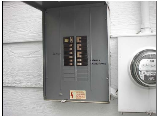
Complete labeling of the main panel is important
