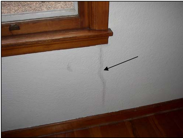
Crack in wall below window of Bedroom 2
