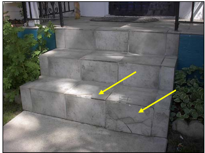
Damaged tile at front step
