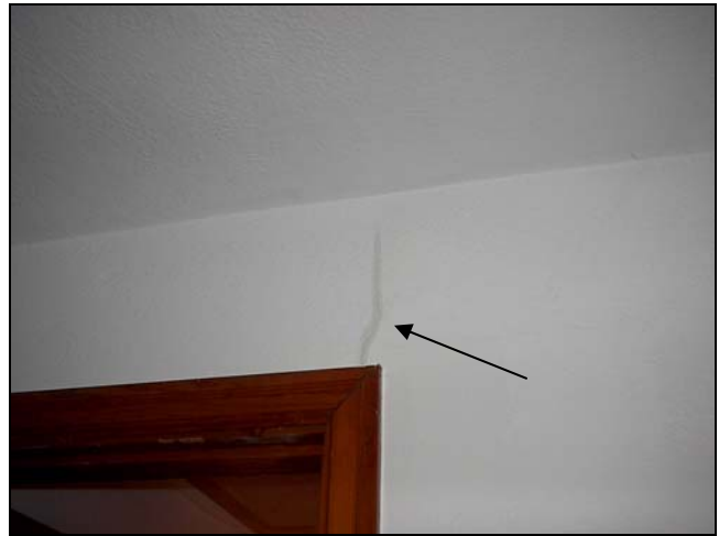
Crack in wall above Bedroom 2 door
