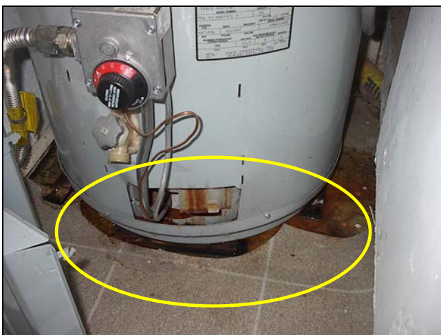
Rust and water leak evident at water heater
