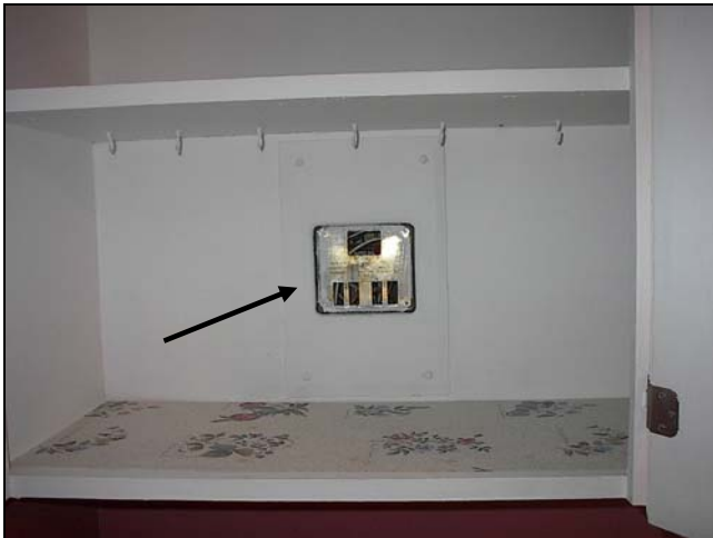
Abandoned panelboard with open slots
