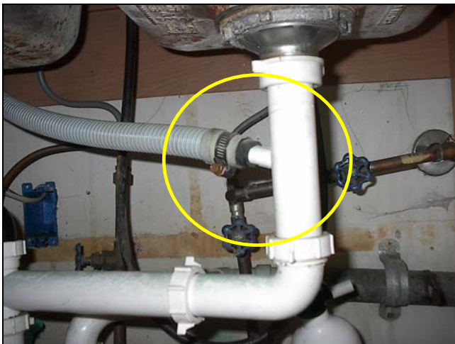
This drain connection is problematic
