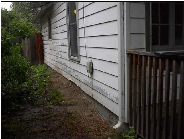
Siding requires priming and re-painting
