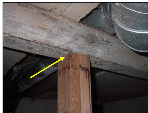
Support post is not properly secured to beam
