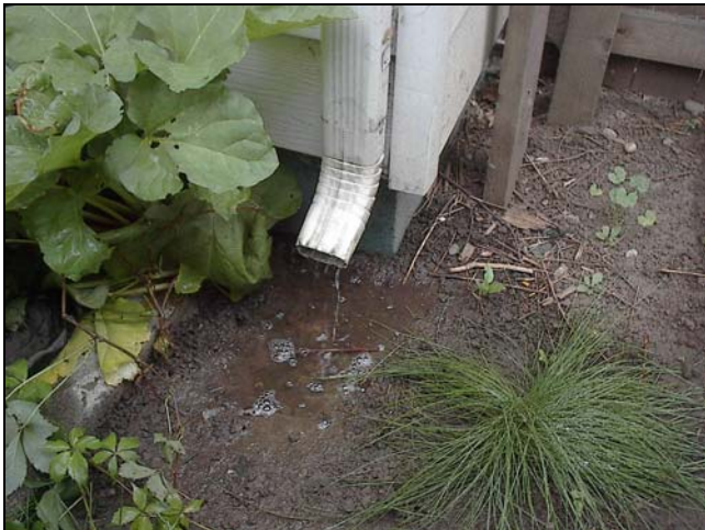
A downspout extension and grading adjustment needed
