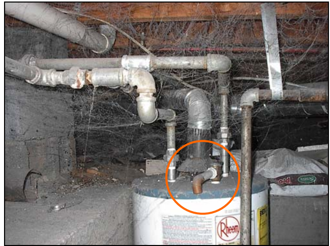
Discharge tube for the water heater is absent
