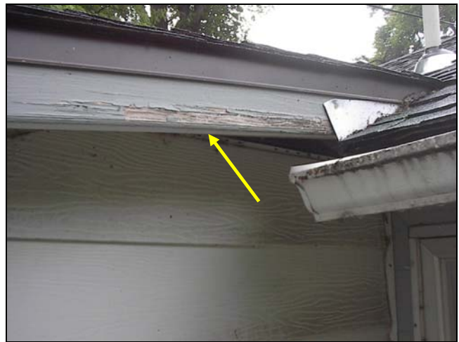
Peeling paint with exposed wood
