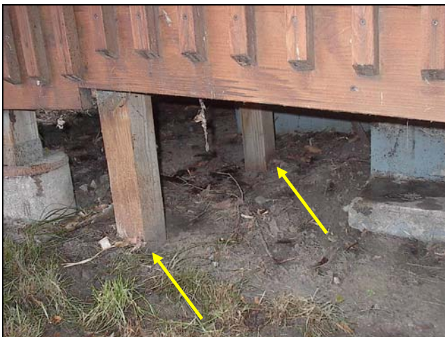
Wood support posts in contact with soil
