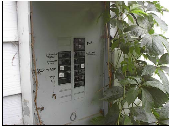
Breakers at panel require complete and accurate labeling
