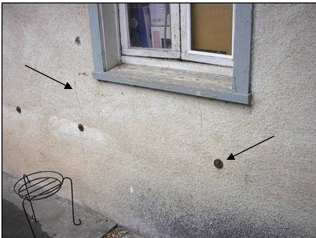
Cracks in exterior walls of garage with supports evident
