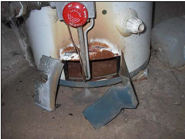
Rust is evident at water heater
