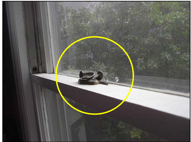
This Bedroom 1 window cannot latch without repair
