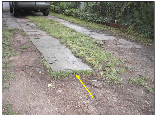
Possible trip hazard
