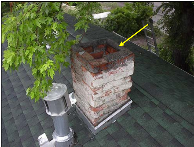
Mortar cap repair and a storm cap is recommended
