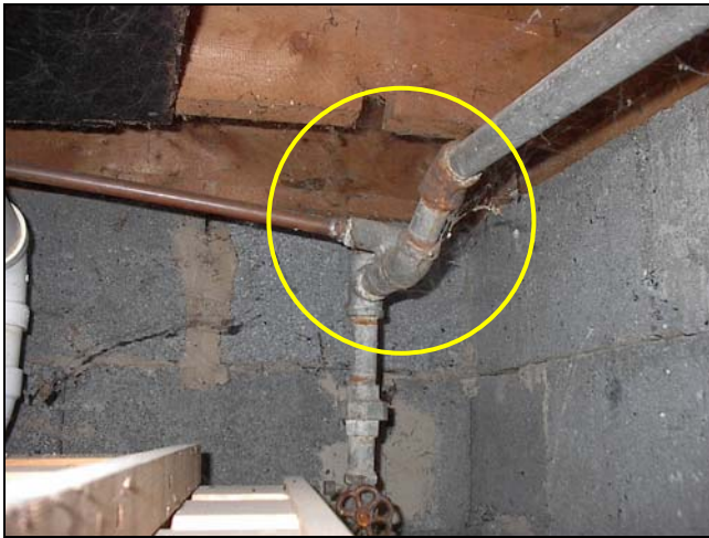
Mixed metals with rust evident near main shut-off valve
