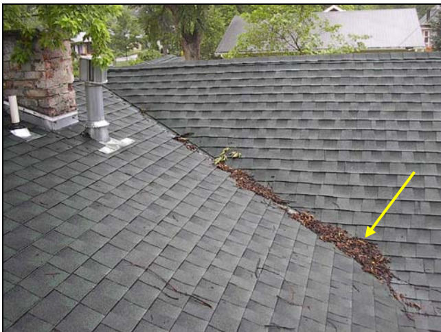
Debris in valley can result in water intrusion into attic
