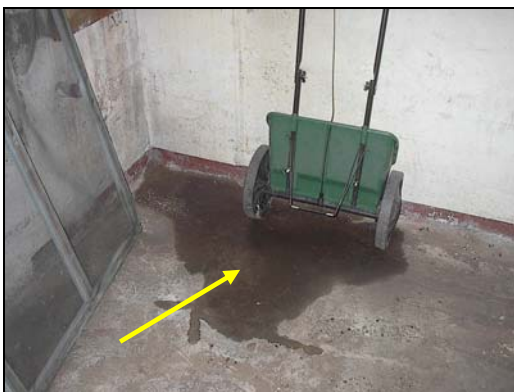
Active water penetration in cellar
