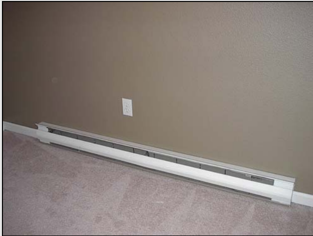
Outlet above family room baseboard heating unit
