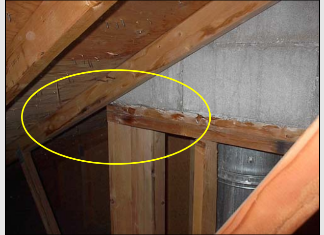
Watermarks on framing member at fireplace chimney
