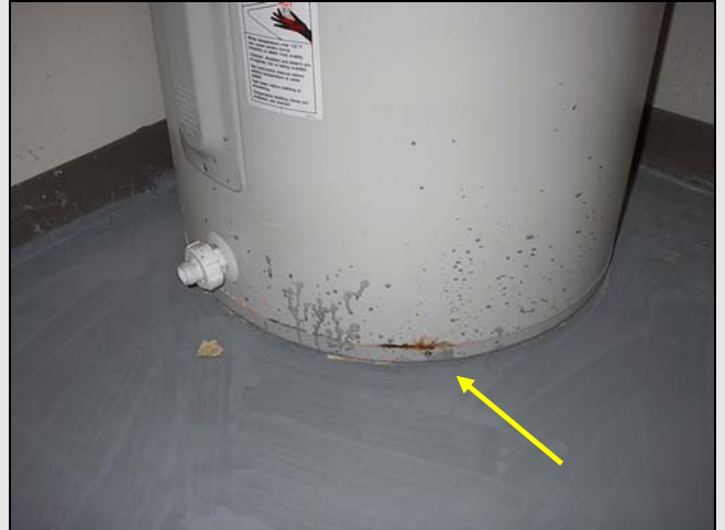
Rust on water heater
