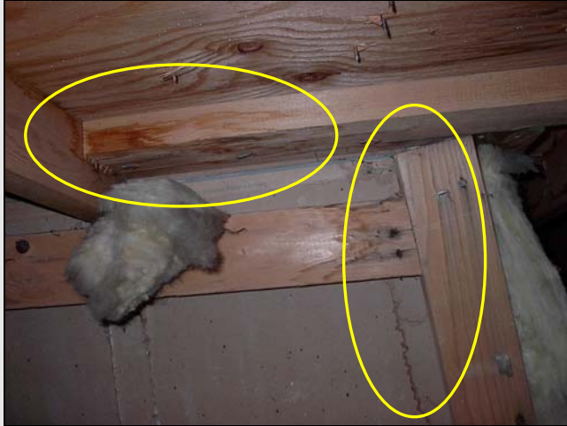
Watermark on framing and skylight well
