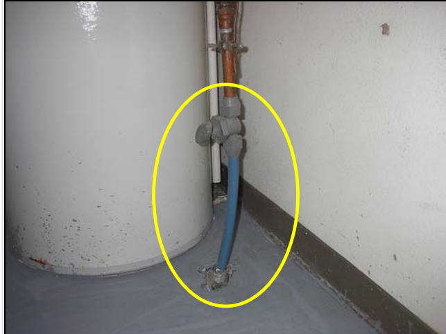
Main water supply line appears to be a polybutylene
