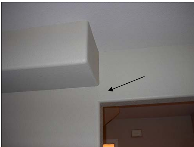
Crack in family room wall
