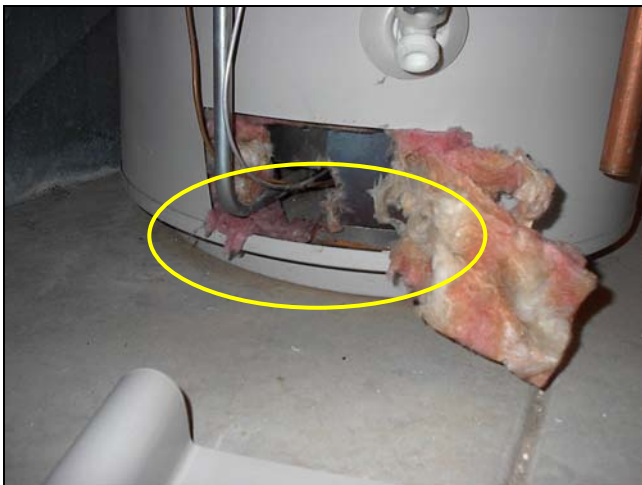
Rust was evident at water heater
