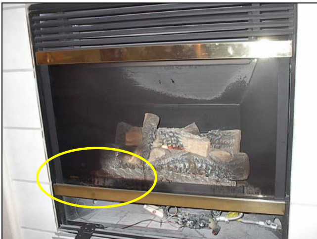
Soot and oxidation evident
