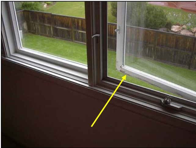
Peeling paint on interior window frame
