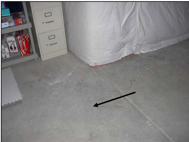
Crack in concrete slab floor
