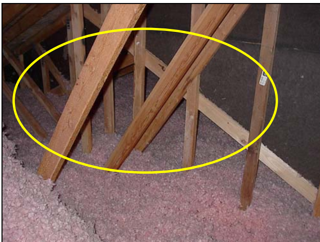
Access to the attic area above Bath 1 was restricted
