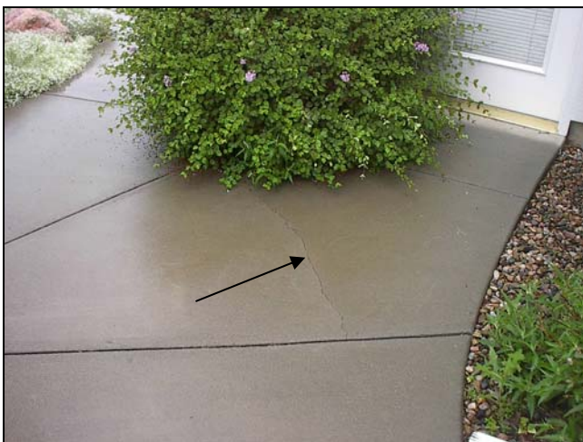
Crack in front walkway
