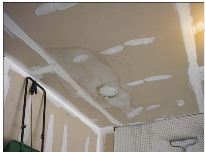
Watermark on garage ceiling
