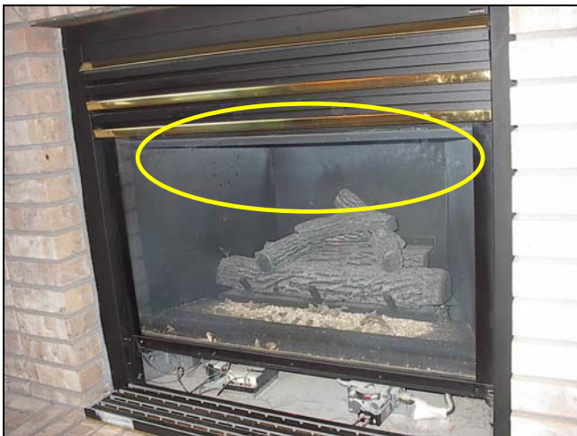
Oxidation on fireplace glass
