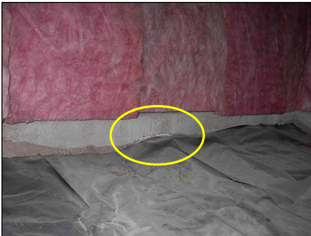
Efflorescence was present on foundation walls
