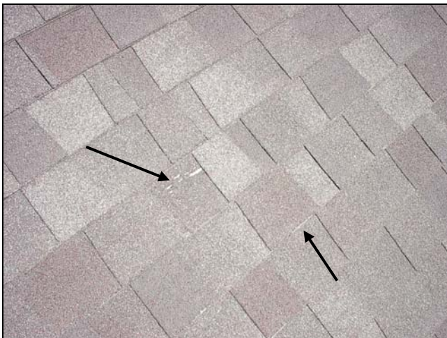
Damage and wear to shingles
