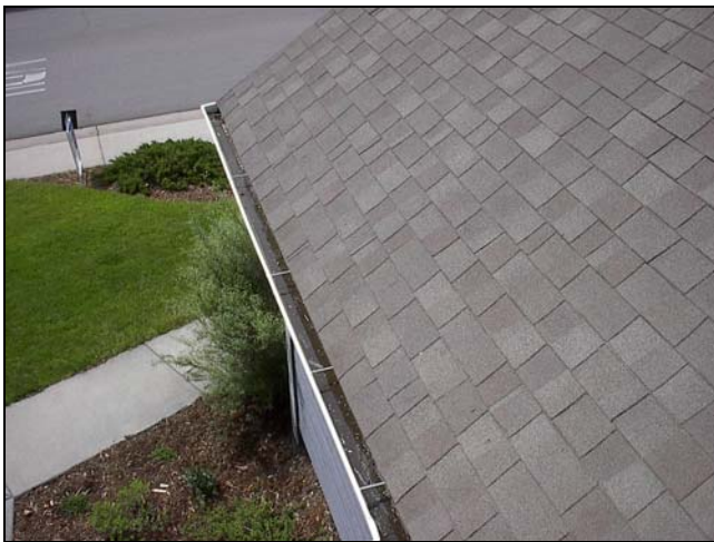
Standing water in east gutter
