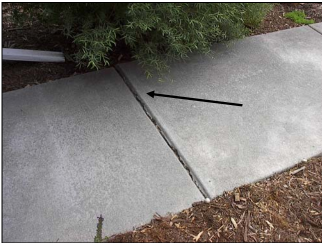
Cracking with displacement
