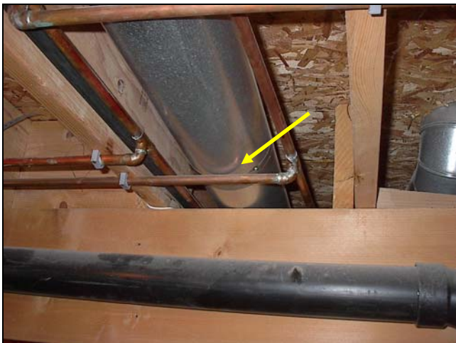
Galvanized metal in contact with copper water supply piping
