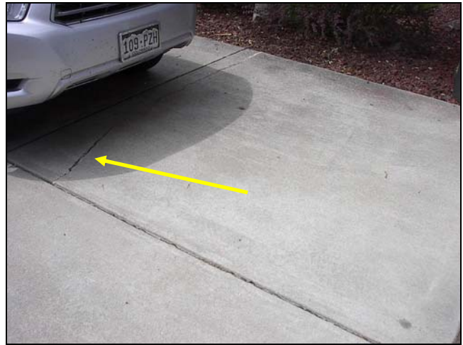
Crack in driveway
