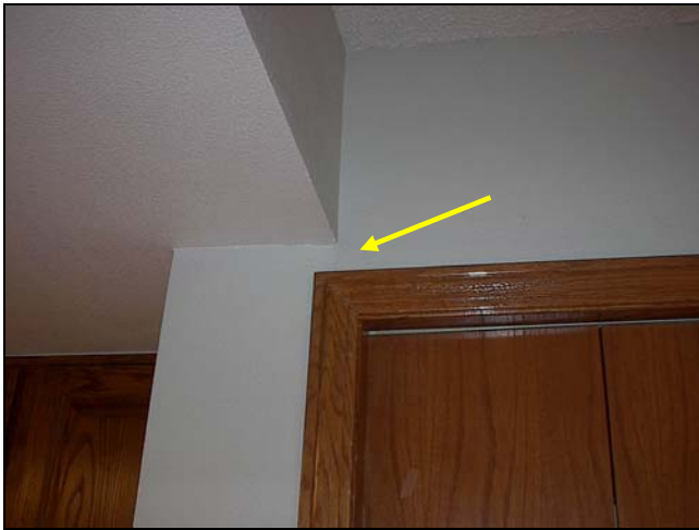
Crack in kitchen wall
