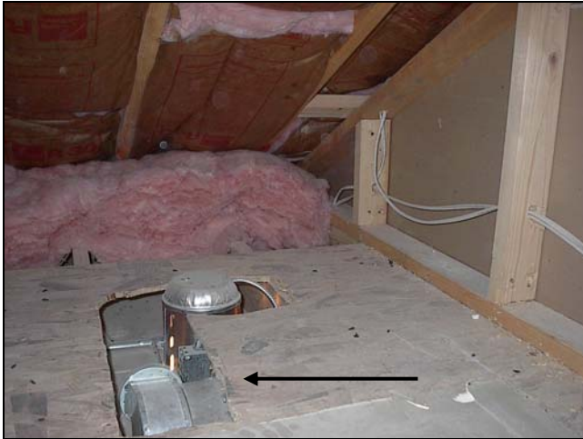
Bath 1 exhaust fan terminates in attic
