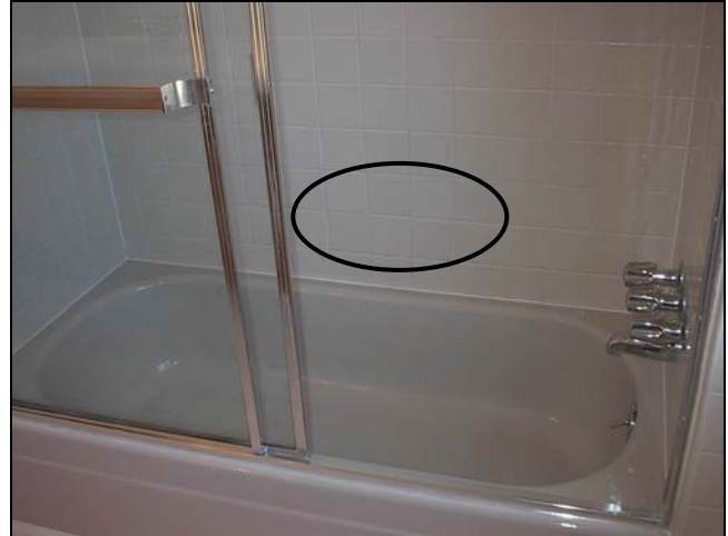
Grout restoration needed
