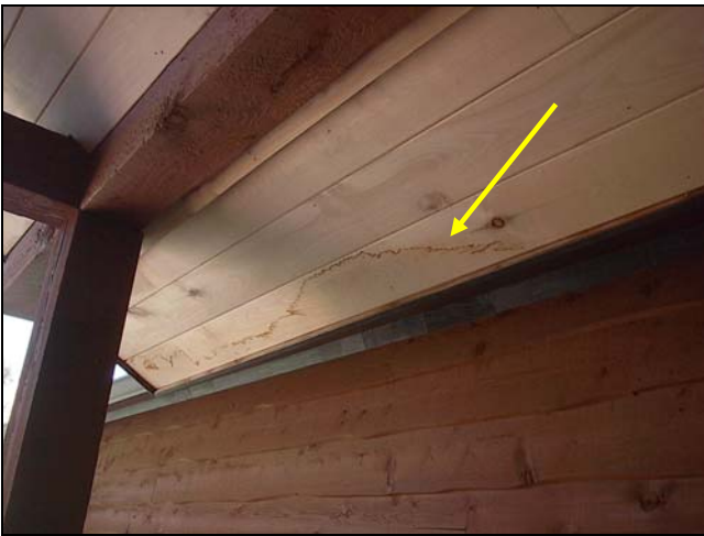
Watermarks on soffit – front porch
