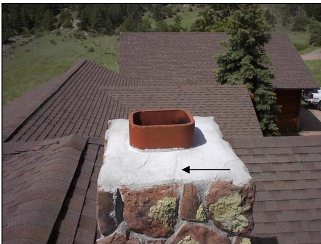
Storm cap needed and cracks in mortar cap (arrow)
