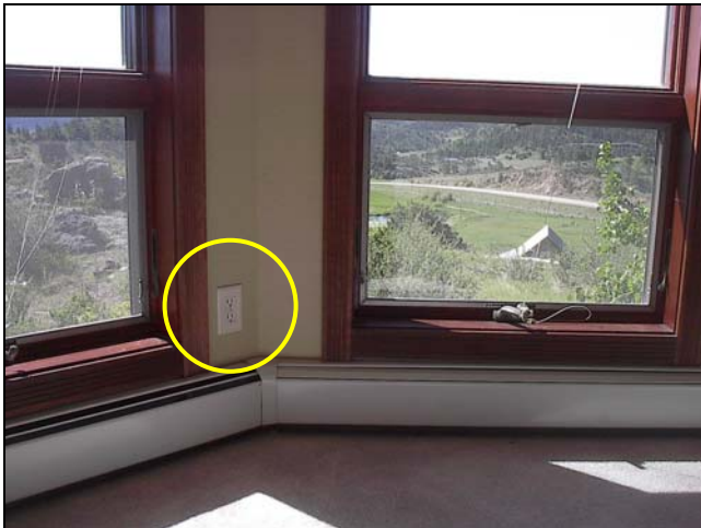
Electric outlet above baseboard heater
