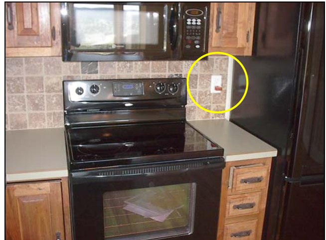
This outlet was not energized
