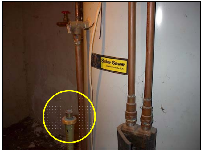
Cut pipe to an apparently abandoned tank
