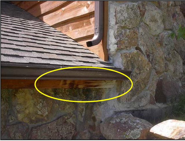
Watermarks on fascia – north
