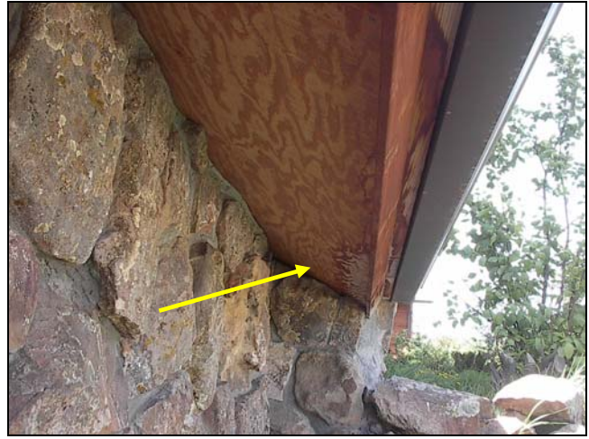
Watermarks on soffit – north
