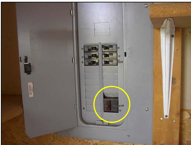
Open slot in main panel
