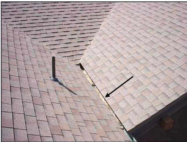
Debris in gutter
