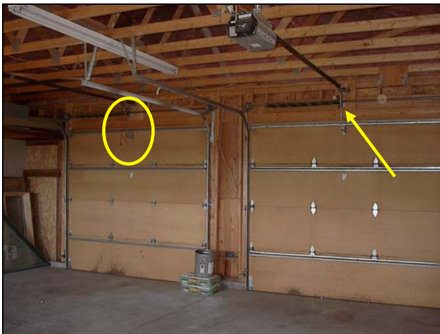
Release handle too high (circle) Release handle missing (arrow)
