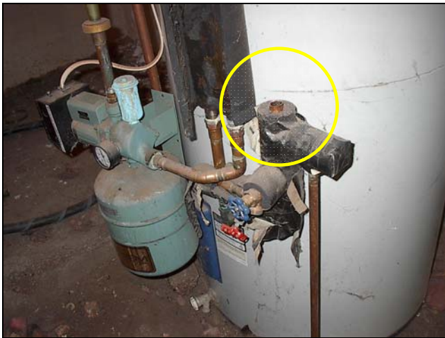
Cut pipe to an apparently abandoned tank
