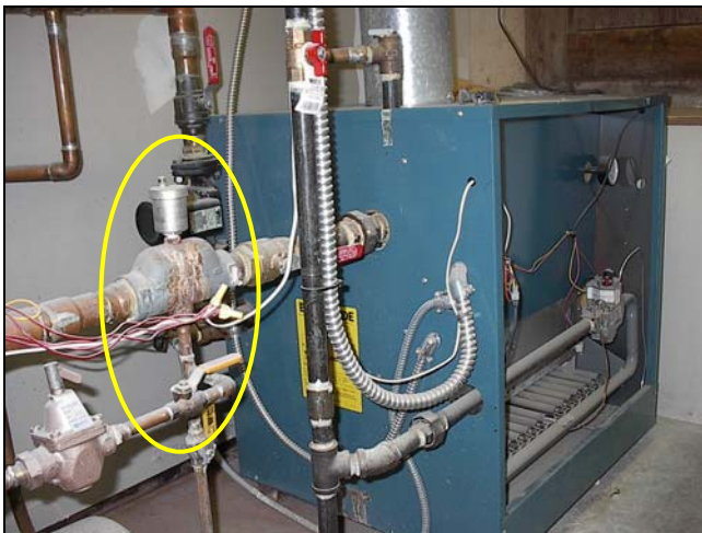
Rust evident at the in-line air vent valve
