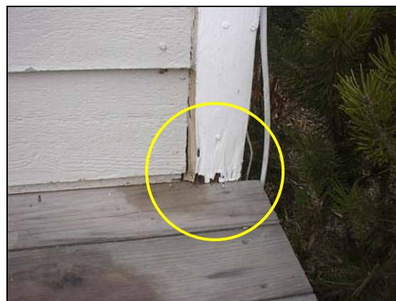
Water damaged wood trim
