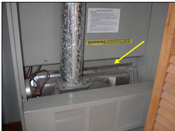
Spillage at induced draft assembly
