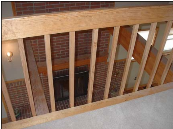
Spacing of guardrail at balcony above living room
