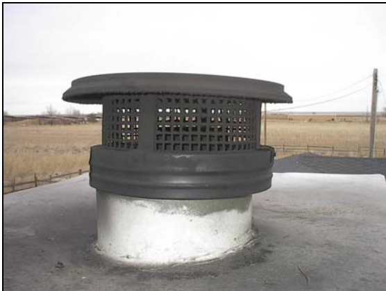
Chimney and chimney caps require cleaning
