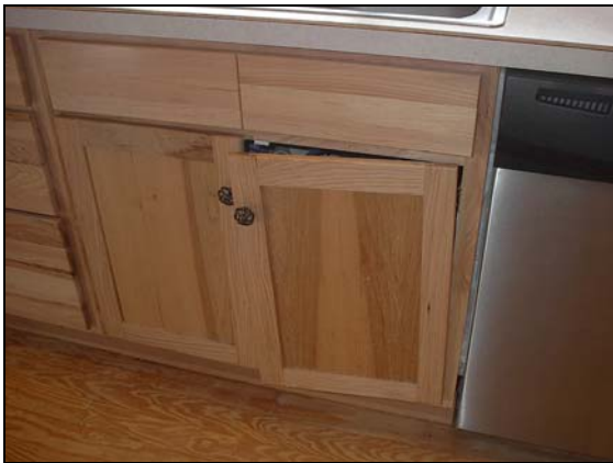
Displaced kitchen cabinet door
