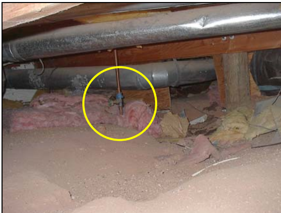
Location of main water shut-off valve
