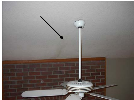
Crack in living room ceiling
