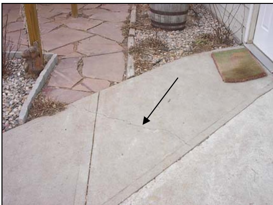
Cracking of walkway
