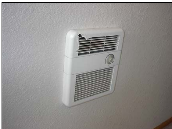
Damaged cover in Bath 1
