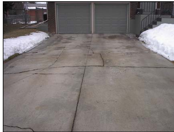
Cracking of driveway
