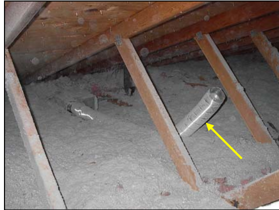
Exhaust duct terminates in attic
