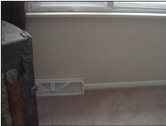
Crack in living room wall
