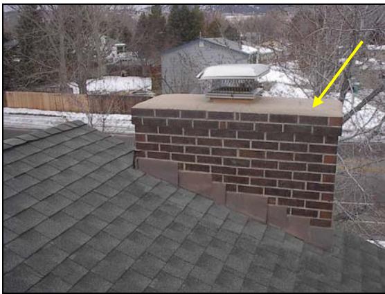
Mortar cap requires caulking
