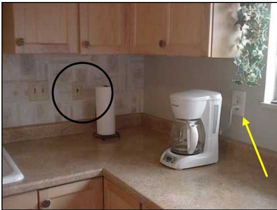
Protected outlet (circle) Unprotected (arrow)
