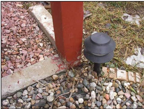
Wood support post (deck) in contact with soil
