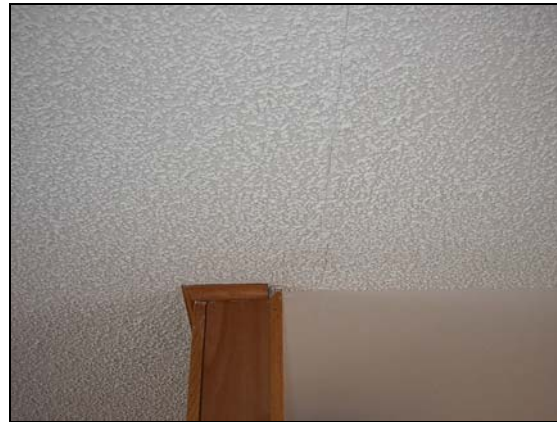
Crack in living room/dining room ceiling
