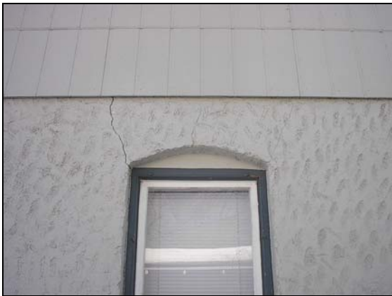
Apparent consequential cracking
