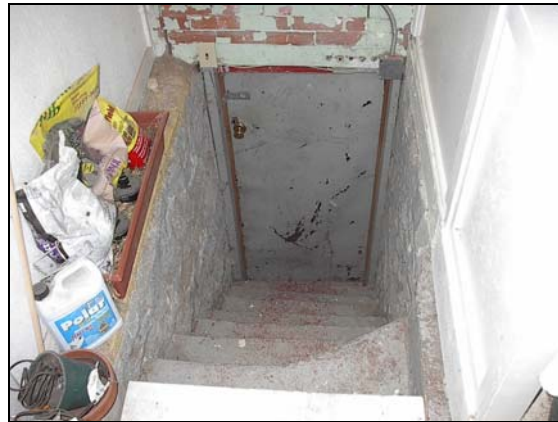
Stairway requires handrail
