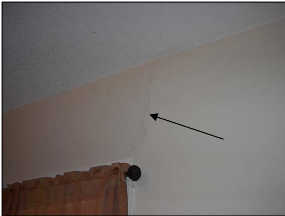
Cracking in Bedroom 1 (main level)
