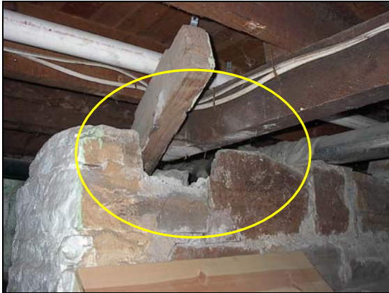
Altered support under main carrying beam
