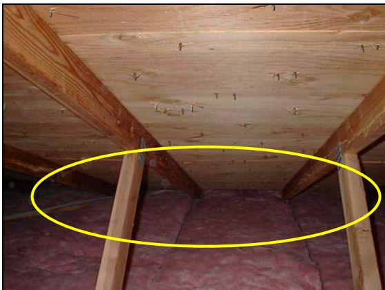
Insulation is preventing proper venting
