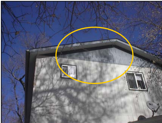
Discoloration of siding
