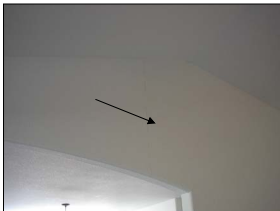
Crack in living room wall
