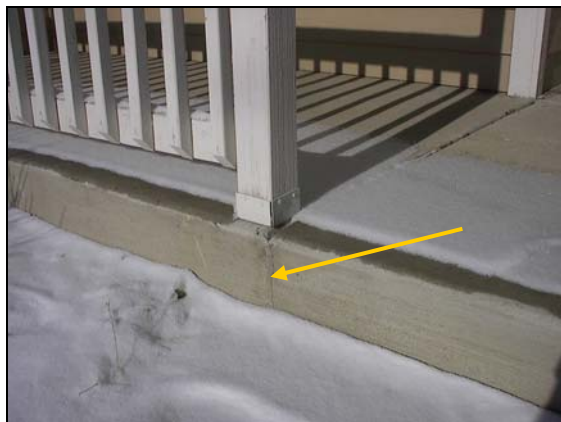
Crack of front porch
