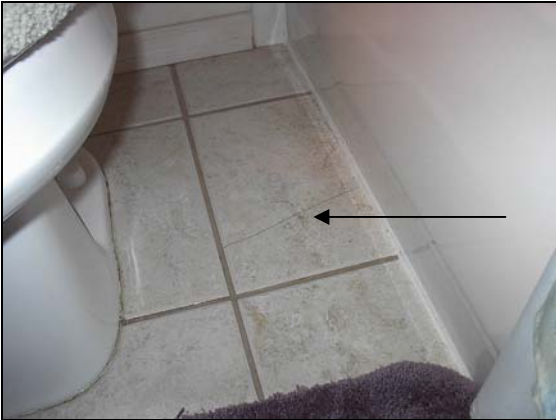
Cracked tile floor in Bath 3
