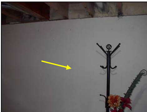
Cracking evident in concrete foundation walls
