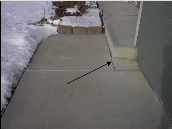
Cracking with displacement of front walkway
