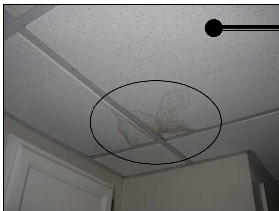
Evidence of previous leak on lower bath ceiling .....
