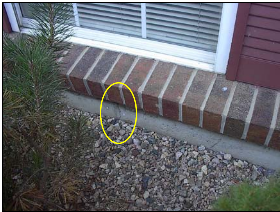
Crack in foundation wall appears inconsequential
