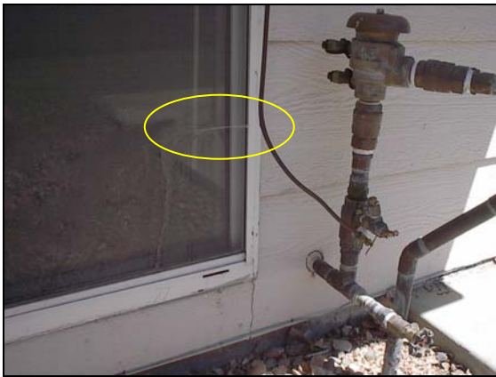
Break in water supply line for A/C unit
