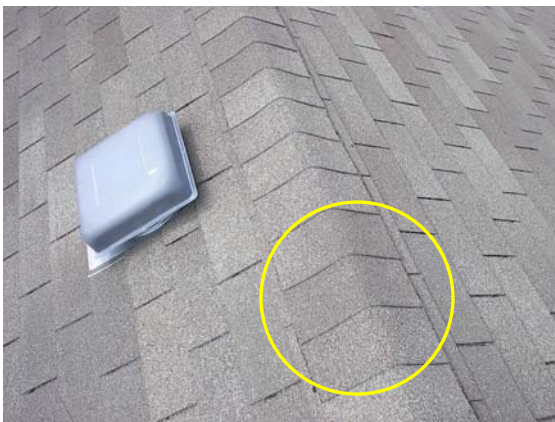
Some cracking of the ridge flashing is evident
