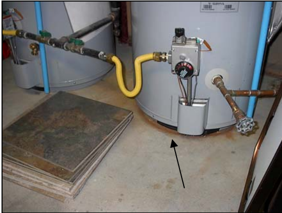
Rust stains appear to be from a prior event and are inconsequential.
