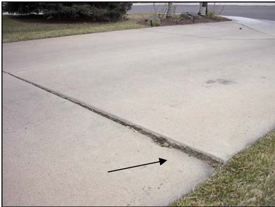
Displacement of driveway
