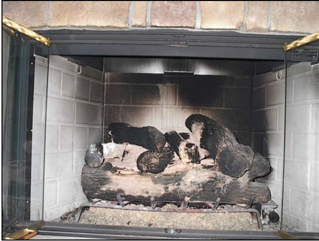
Soot on log set and fire chamber
