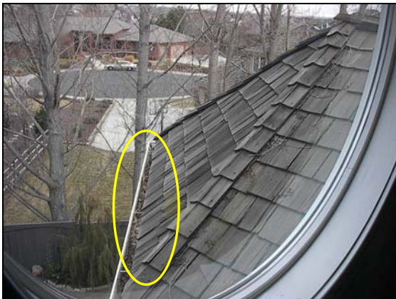
Gutters require cleaning
