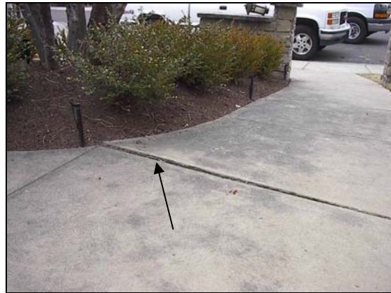
Displacement of front sidewalk
