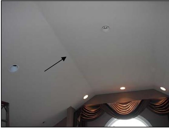
Living room ceiling displays cracking
