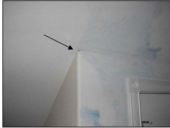
Cracking in exercise room
