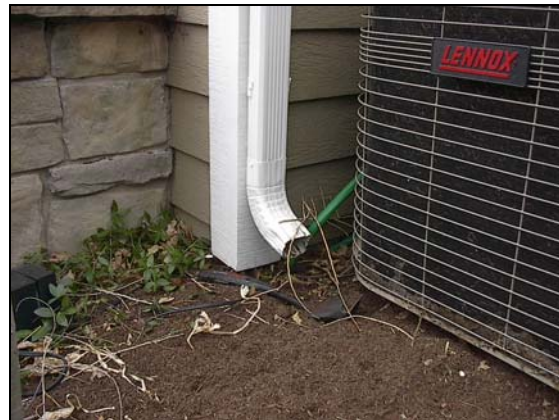
This downspout requires an extension
