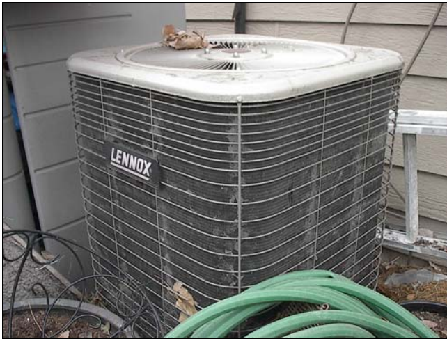
Condenser fins of System #2 exterior condenser require cleaning
