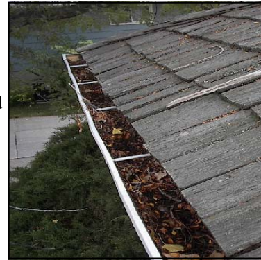
Clogged gutters create problems
